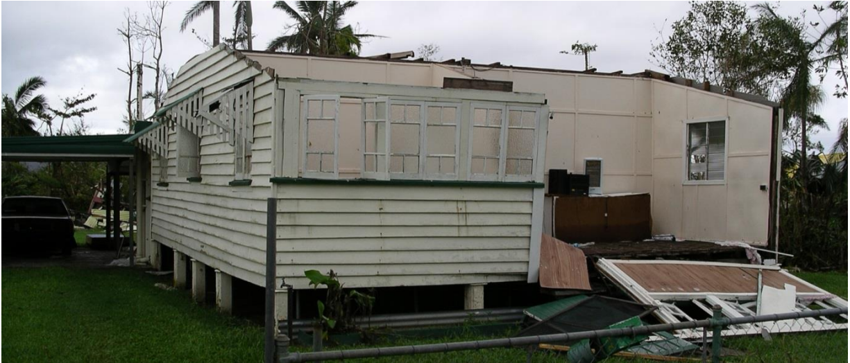
Figure 15. Roofing and wall damage to a low-set 1930s home as presented to builders, assessors, and engineers for experience based estimates of repair cost (high-set costs were also evaluated)
