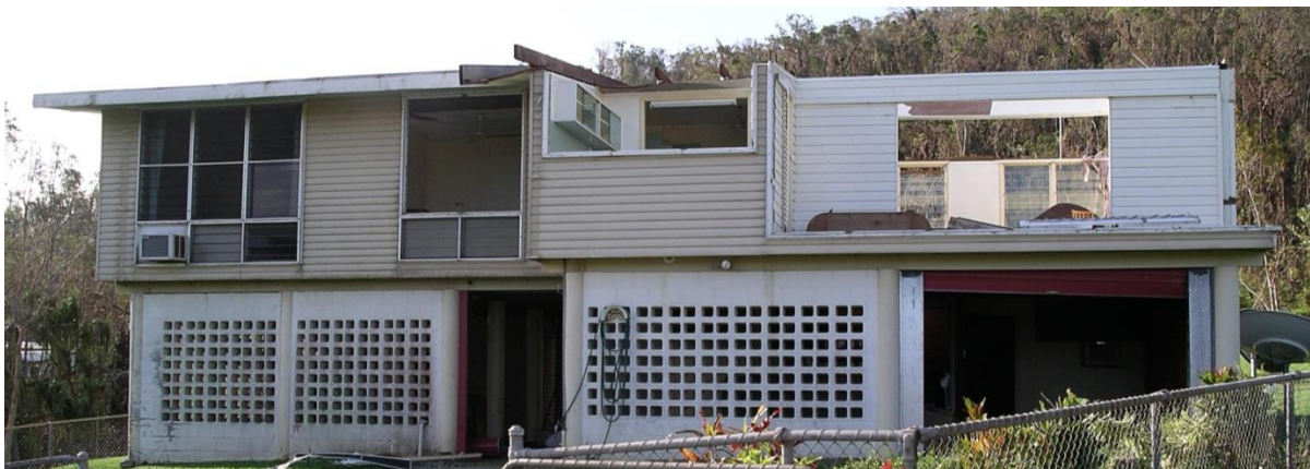
Figure 16. Roofing and wall damage to a high-set 1970s home as presented to builders, assessors, and engineers for experience based estimates of repair cost
