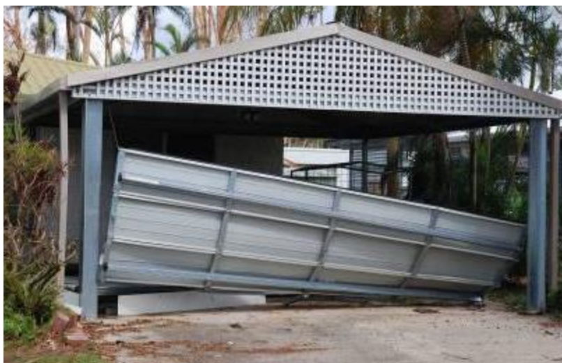
PICTURE 3-2 – OPENINGS DAMAGE
