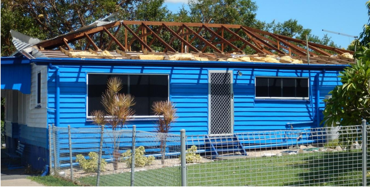
Figure 12. Wind-induced roofing damage to a low-set 1930s home as presented to builders, assessors, and engineers for experience based estimates of repair cost
