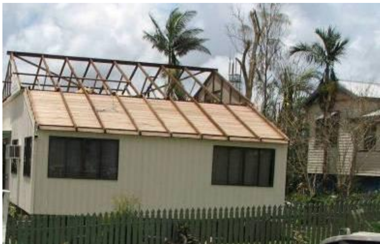
PICTURE 3-1 – ROOFING DAMAGE
