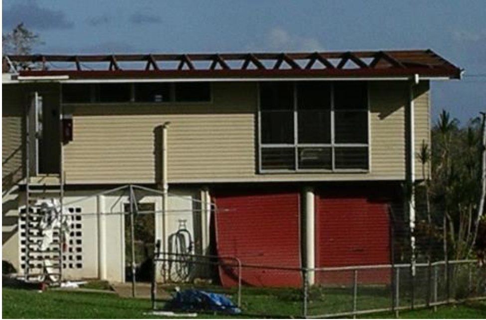
Figure 13. Wind-induced roofing damage to a high-set 1970s home as presented to builders, assessors, and engineers for experience based estimates of repair cost
