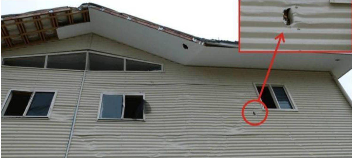
Figure 14. Wind driven debris damage to a modern home as presented to builders, assessors, and engineers for experience based estimates of repair cost
