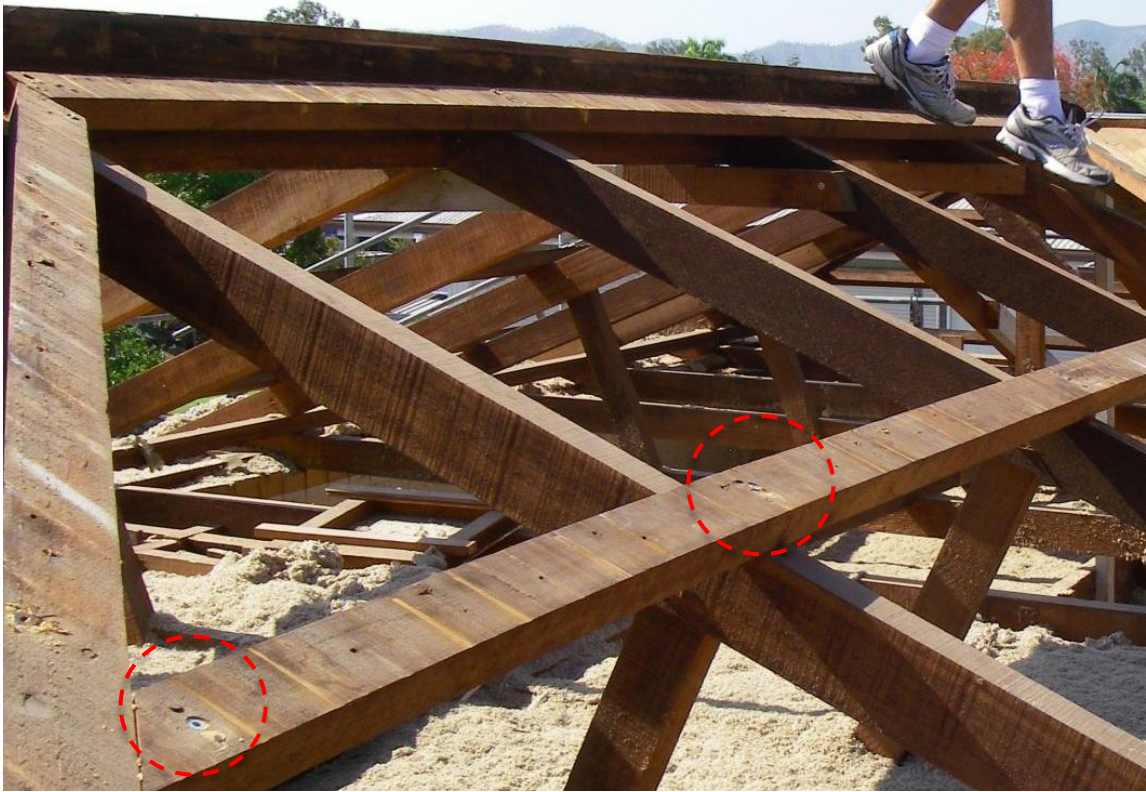
Figure 17. Batten screw from battens to rafters (pre drill before installing batten screws)
