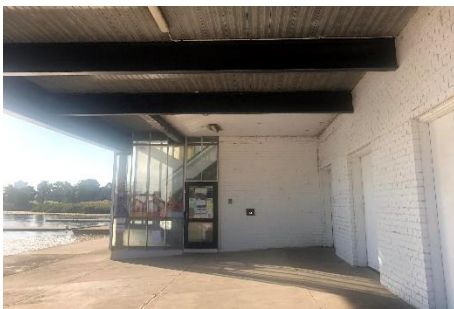
Current entry is uninviting and poses a major barrier for engagement for many different user groups. It also lacks any accessible entry.
