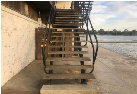
Stair access available on the exterior of the building is timber planks on top of metal frame with timber treads and bolts now requiring monthly inspection and maintenance.
