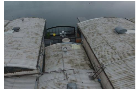
The construct of the roof curved with rusting gutters and the roof itself has been deemed unsafe for standard trade access to repair due to its age and asbestos material.
